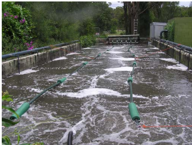
Sewerage Treatment tank with air stone aeration installed.
