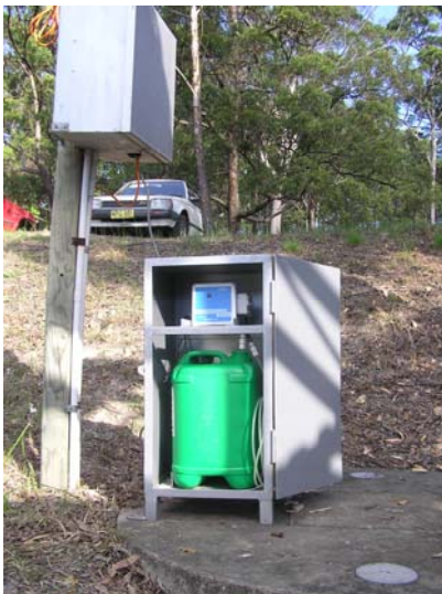
Automated Septic dosing
