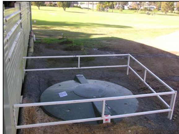
Collection tank, water pumped to separator.
