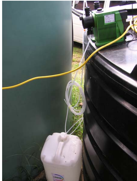
Automatic dosing of Odour Kill into irrigation line
