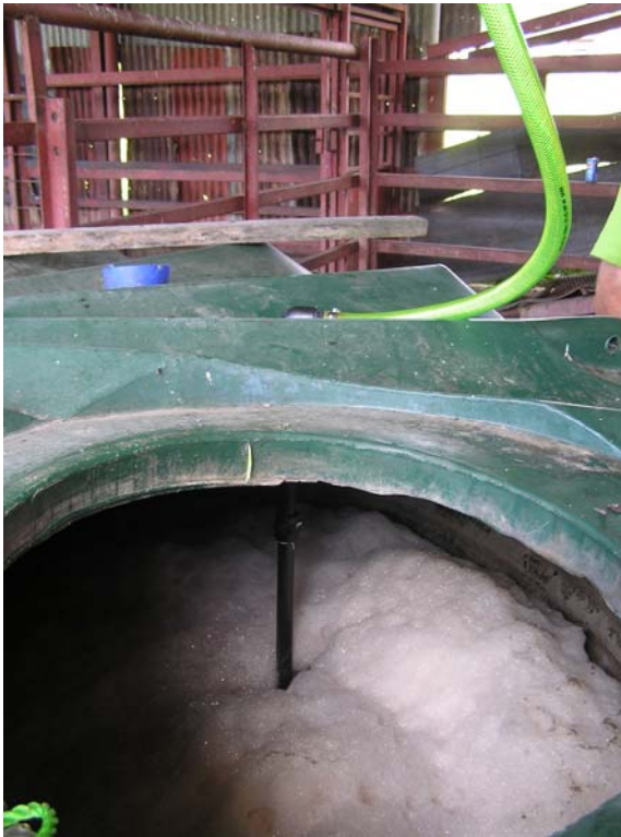
Tank aeration & Bio Plus
