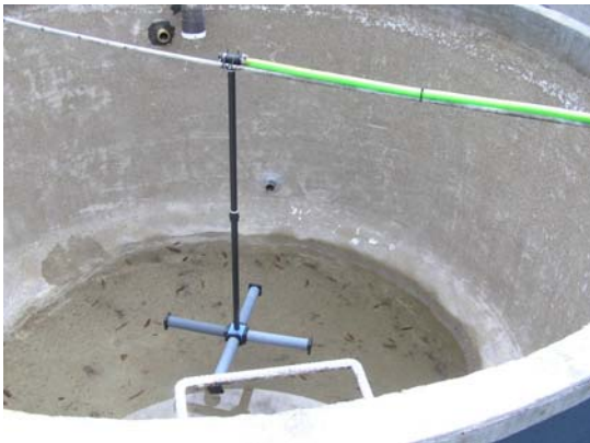
Tank aeration & Auto dosing
