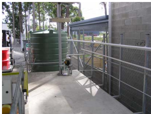
Holding tank for decanted water
